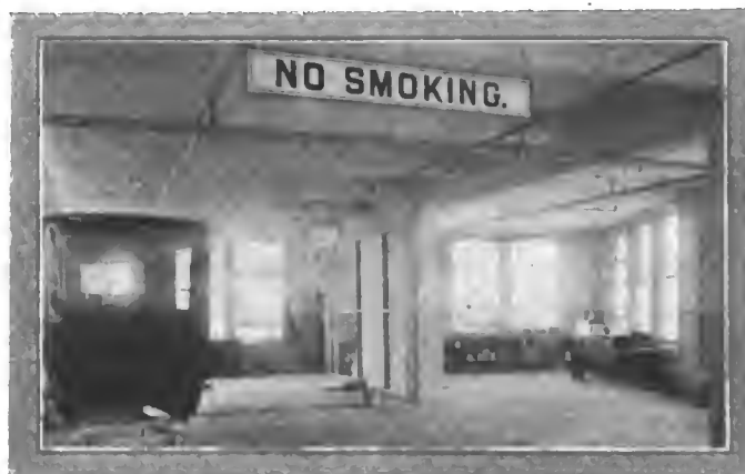
9—Where the body work is done: a dust-proof varnishing room partly finished is shown at the left
